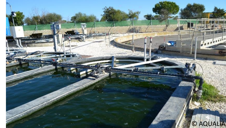
High Rate Algae pond systems in Chiclana wastewater treatment plant, operated by AQUALIA in Spain, for bio-plastics production, © AQUALIA
