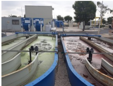
High-Rate Algae Ponds in Chiclana, during the aeration phase © AQUALIA
